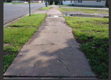
This deteriorated sidewalk is located on Madison Street between North 13 th Street and North 14 th Street. Note the water standing on the sidewalk.
