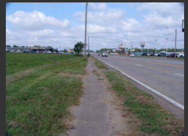
This sidewalk is deteriorating along Park Avenue near Paducah Ford.
